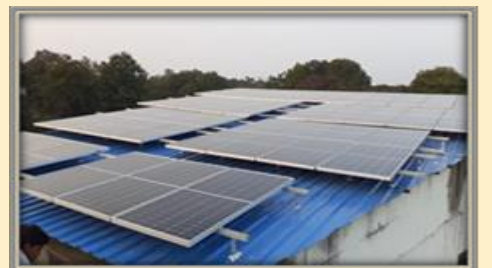
Solar Power Plant 26KW Capacity
